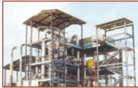
Solvent Extraction Plant
